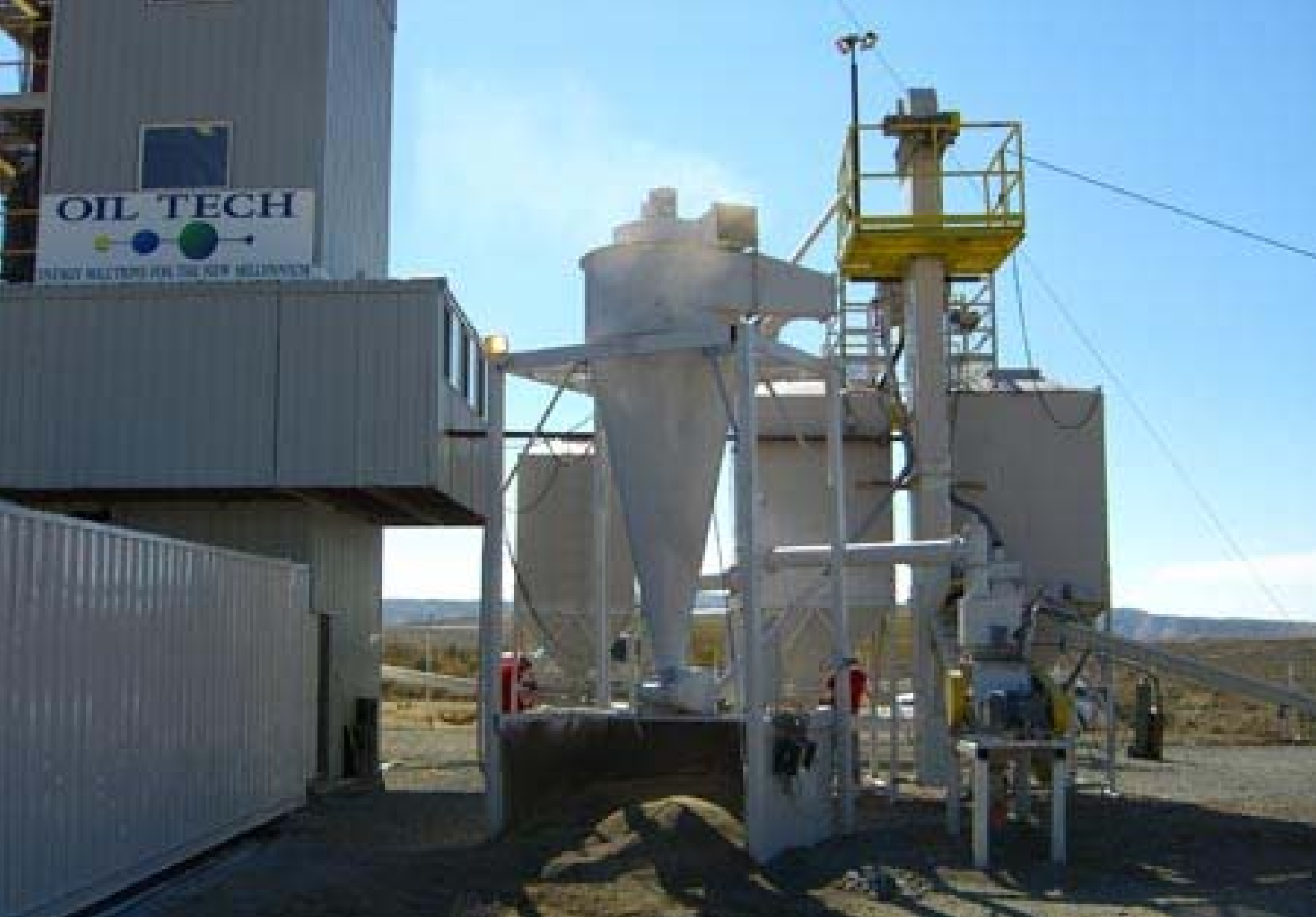
Dust Collector & Rock Processing Equipment
